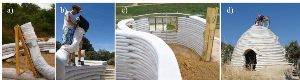
Figure 1: Construction of superadobe structures (sources: www.labioguia.com (a), www.domoterra.es (b, d), www.earthbagbuilding.com (c)).
