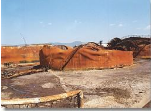
Figure 1: Damaged Liquid Storage tank (A) due to sloshing, Ref Carleton University
