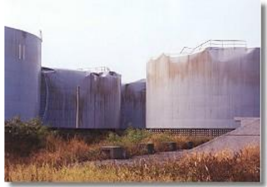
Figure 2: Damaged Liquid Storage tank (B) due to sloshing Ref: Carleton University
